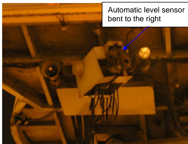
Figure 3. Damage to aerobridge automatic level sensor
